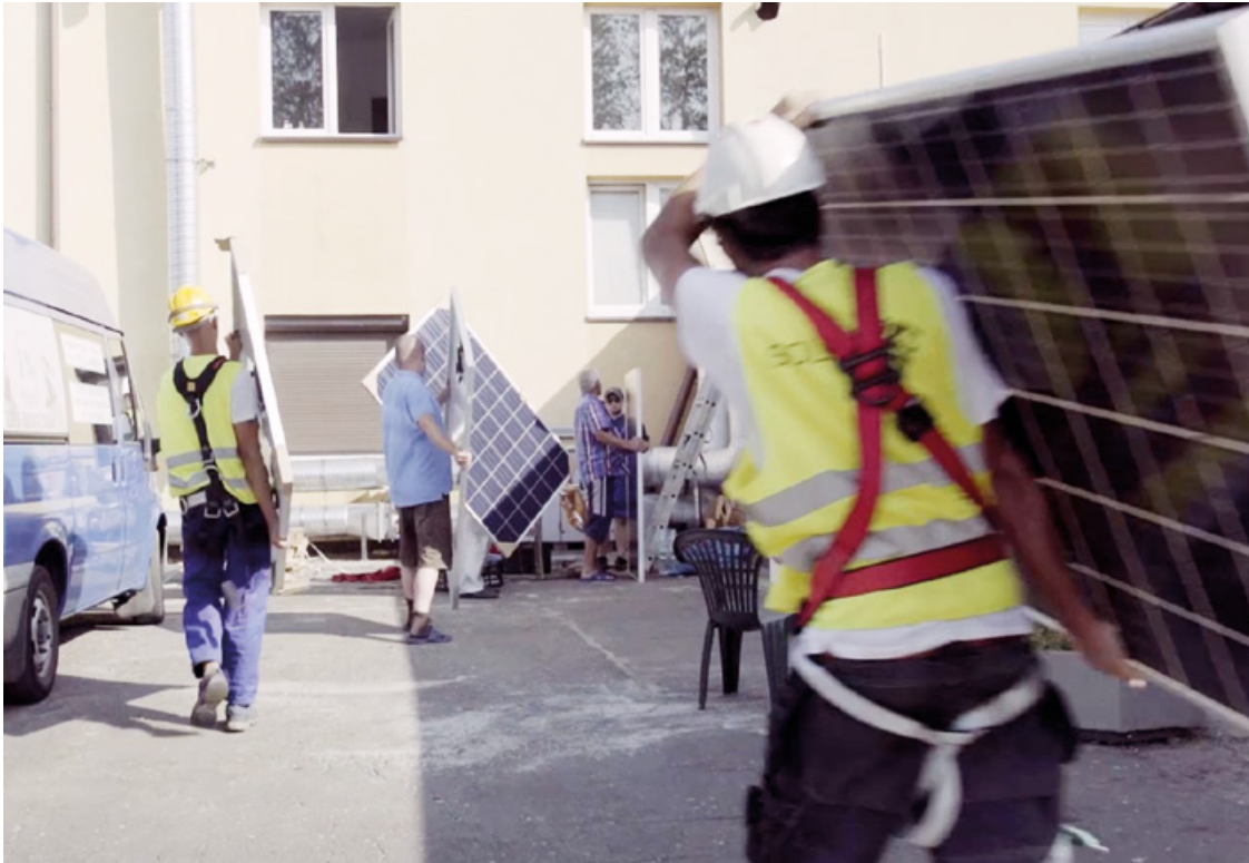
Mounting of the PV installation on the rooftop of the homeless shelter in Słupsk.
