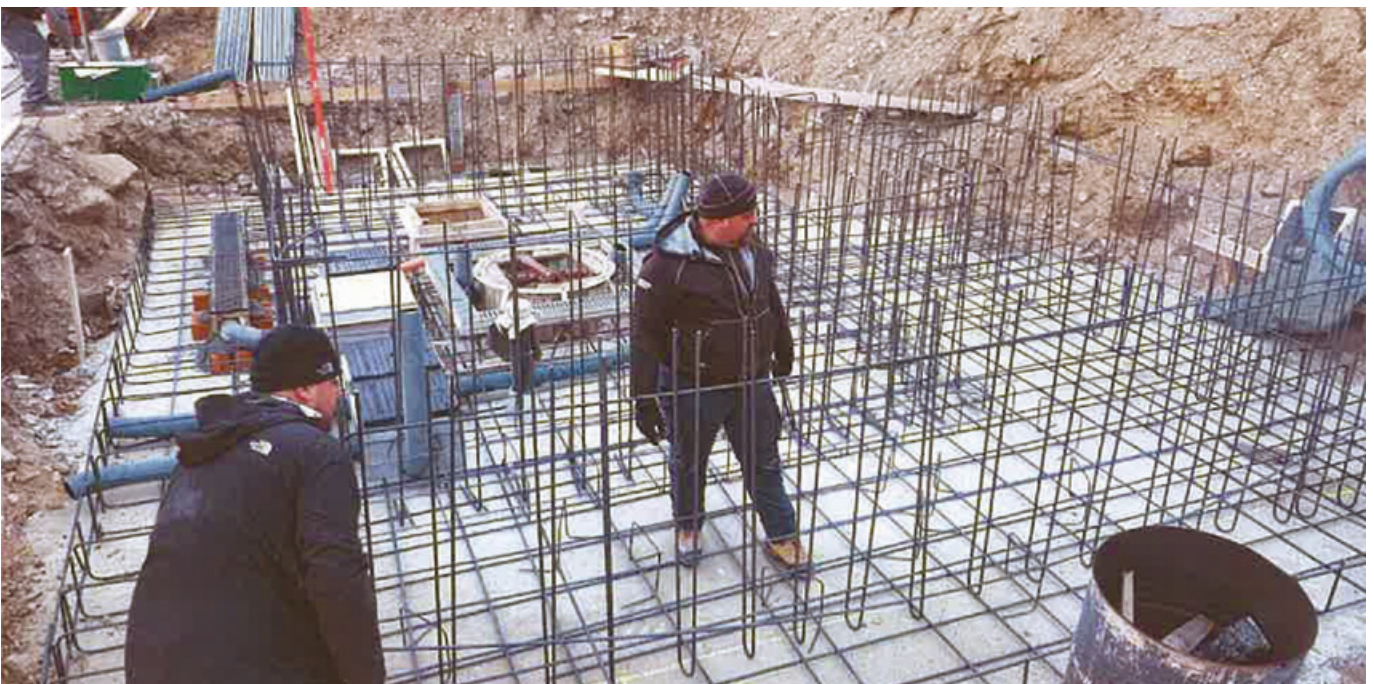
Construction site of the Venaus hydro-power plant in the Susa Valley, Italy.
